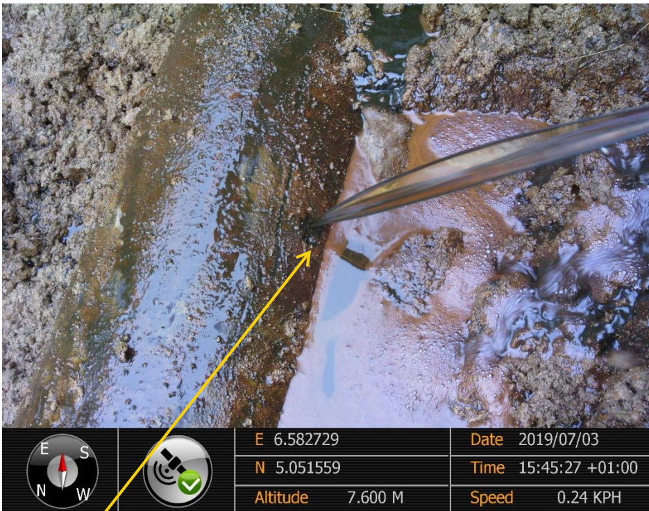
Close-up: Drilled Hole on 14" Okordia - Rumuekpe Pipeline at Ula-Ikata. Picture was taken during Joint Investigation of 3 rd July 2019
