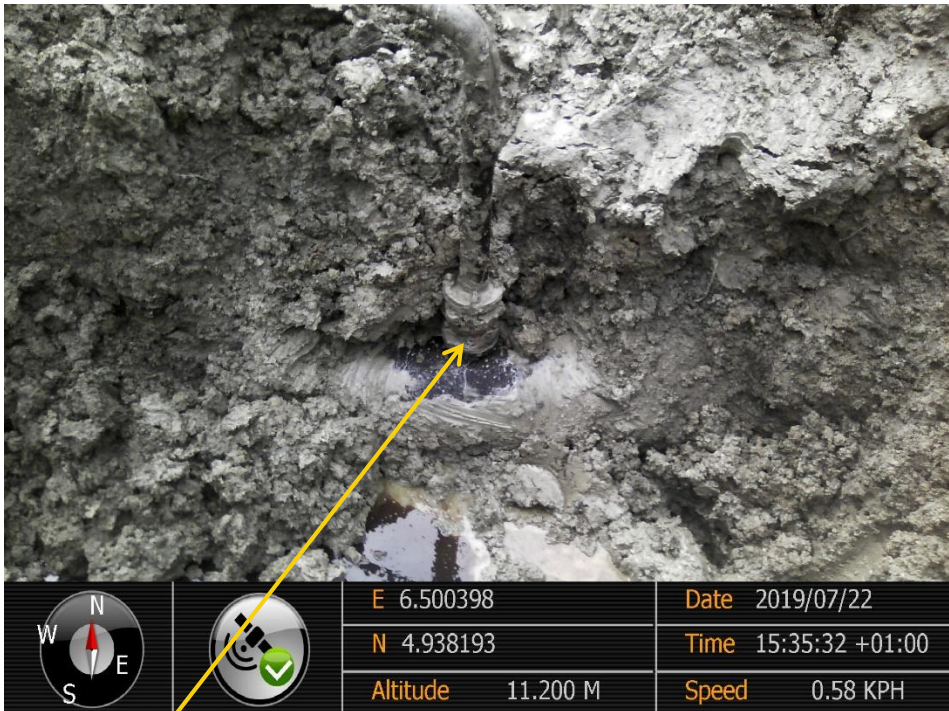
Close-up: Illegal fitting on 20'' Kolocreek - Rumuekpe Pipeline at Odau-km19. Picture was taken during Joint Investigation of 22 nd July 2019.
