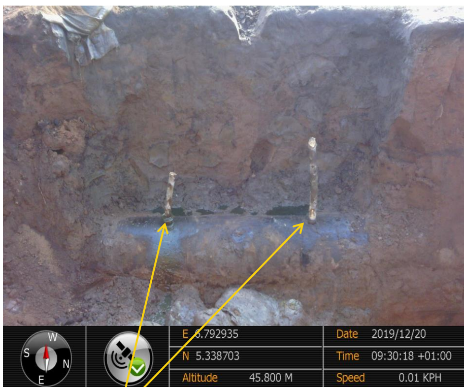
Close-up: Plugged illegal fittings on 18" Assa - Rumuekpe Pipeline at Assa. Picture was taken during Joint Investigation of 20 th December 2019.
