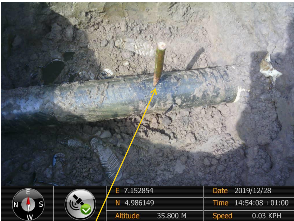
Close-up: Plugged Drilled Hole on 8" Nkali - Imo River 2 Pipeline at Odagwa . Picture was taken during Joint Investigation of 28 th December 2019.
