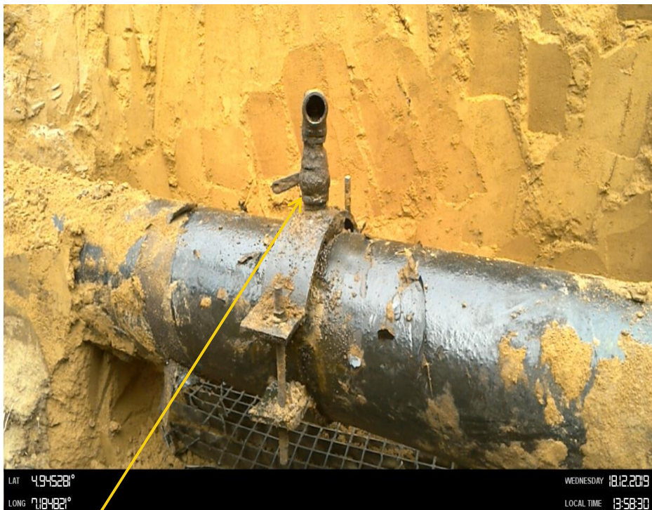
Close-up: Illegal fitting on 12" Imo River2 Pipeline at Umuololo . Picture was taken during Joint Investigation of 18 th December 2019.
