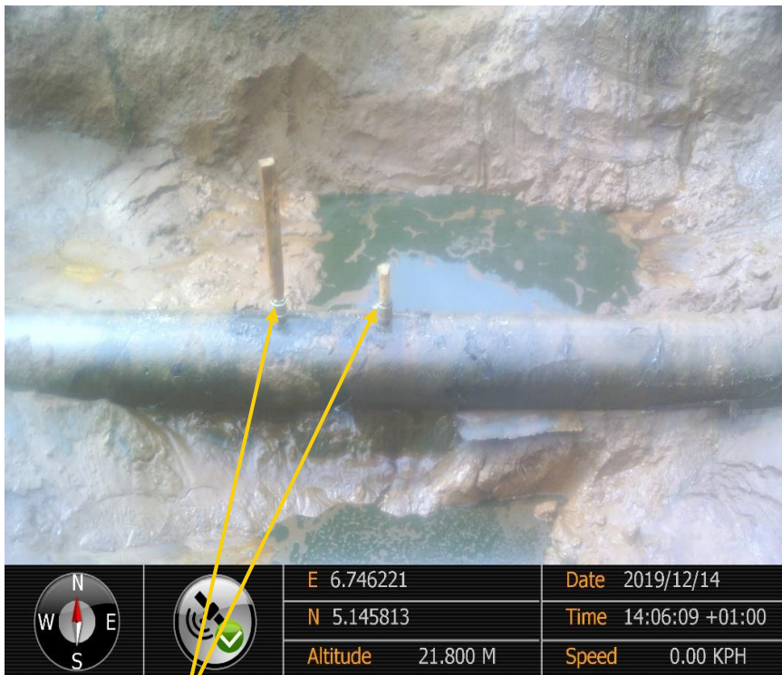
Close-up: Plugged illegal fittings on 18inch Assa Rumuekpe Pipeline at Umudioga/Akpabu. Picture was taken during Joint Investigation of 14 th December 2019.
