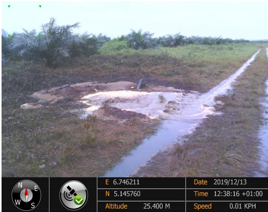
Overview: Part of spill impact on 18inch Assa Rumuekpe Pipeline Right of Way at Umudioga-Akpabu. Picture was taken during Joint Investigation of 13 th December 2019.
