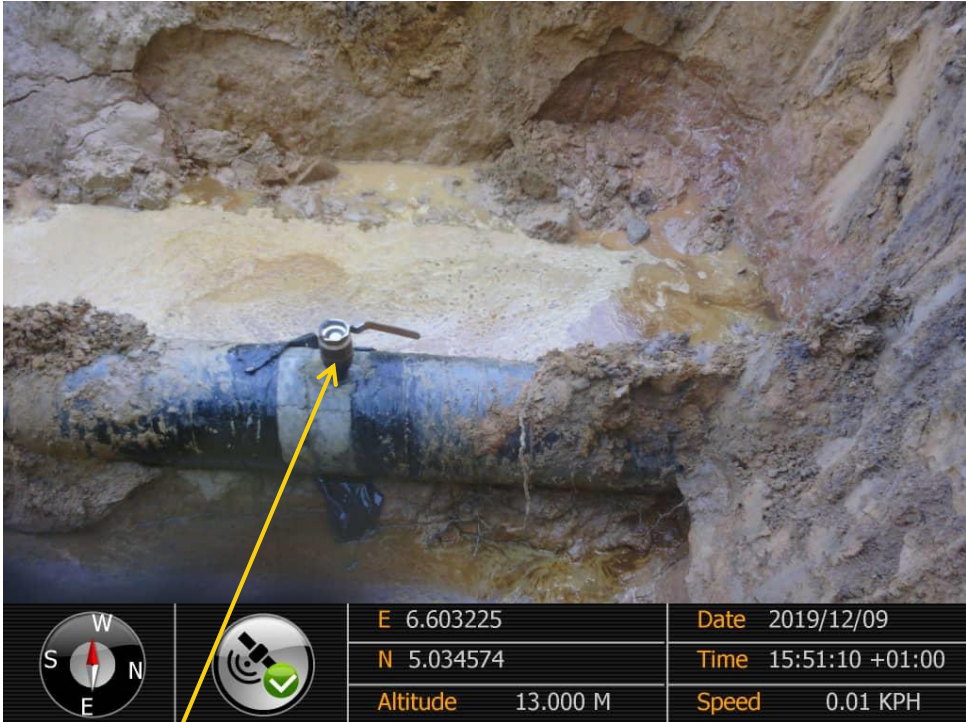
Close-up: Illegal Fitting on 14" Okordia – Rumuekpe Pipeline at Ikata . Picture was taken during Joint Investigation of 9 th December 2019.
