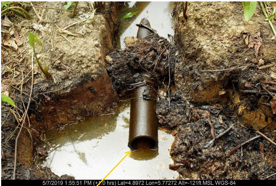
Close-up: Missing part of the Flowline on 4" Opukushi Well 33L/S Flowline at Egbemo-Analabiri-agbidiana. Picture was taken during Joint Investigation of 7 th May 2019.
