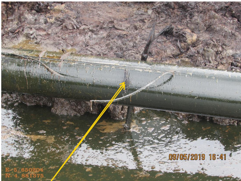
Close-up: Hack Saw Cuts on 6'' Tunu Kanbo Well 7L Flowline at Egbemo-Analabiri-agbidiana. Picture was taken during Joint Investigation of 9 th May 2019.
