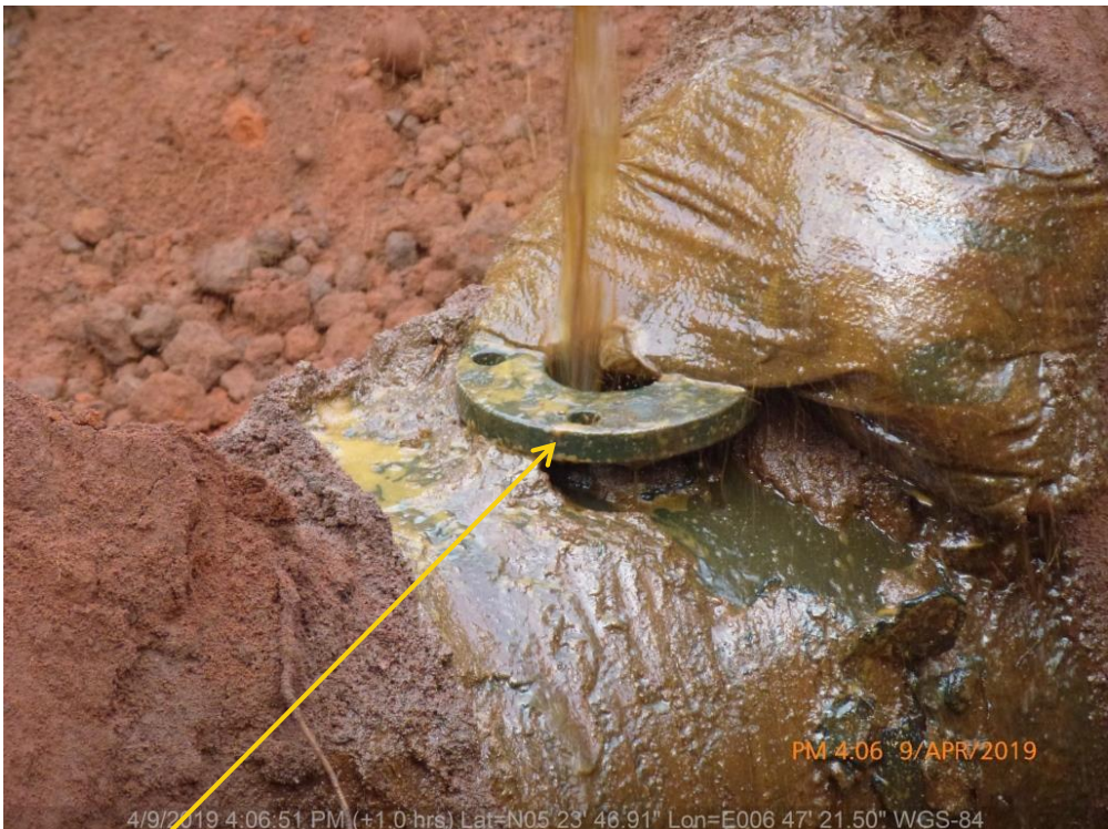
Close-up: Illegal fitting on 16" Egbema - Assa Pipeline at Obile. Picture was taken during Joint Investigation of 9 th April 2019
