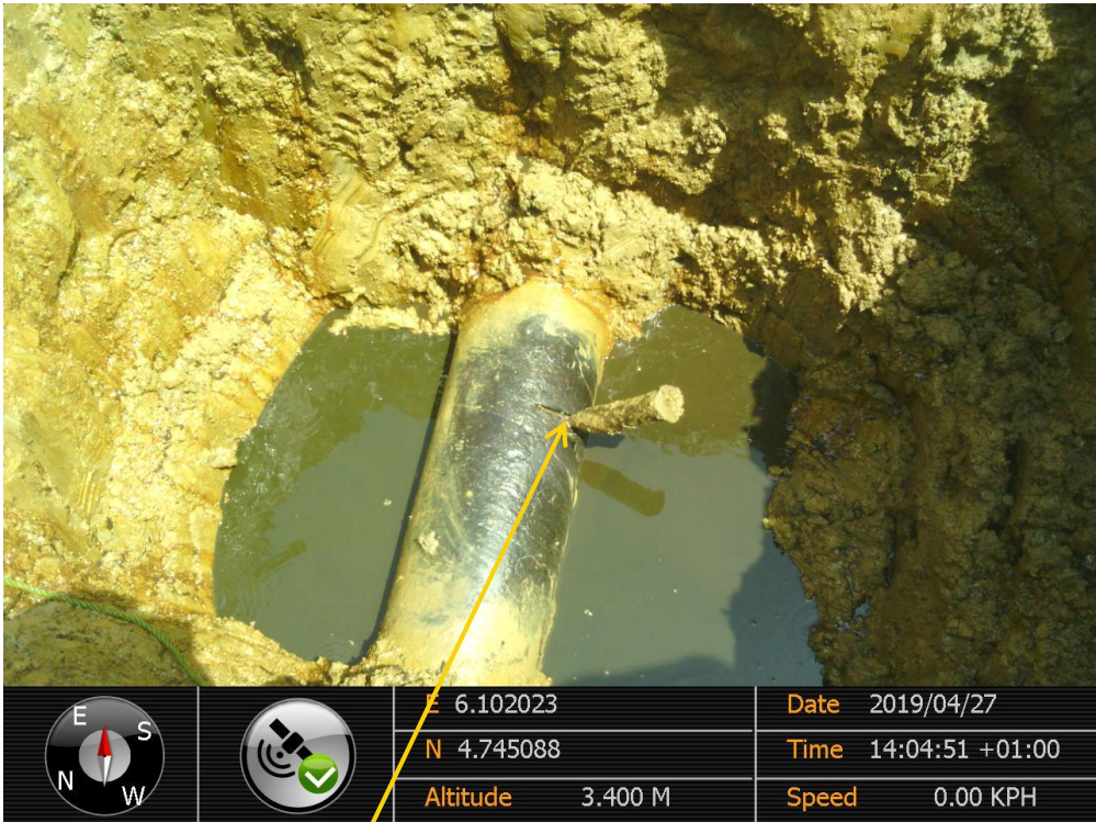
Close-up: Plugged Hack Saw Cut on 10" Diebu – Nunriver Pipeline at Onyoma / Ekowe. Picture was taken during Joint Investigation of 27 th April 2019
