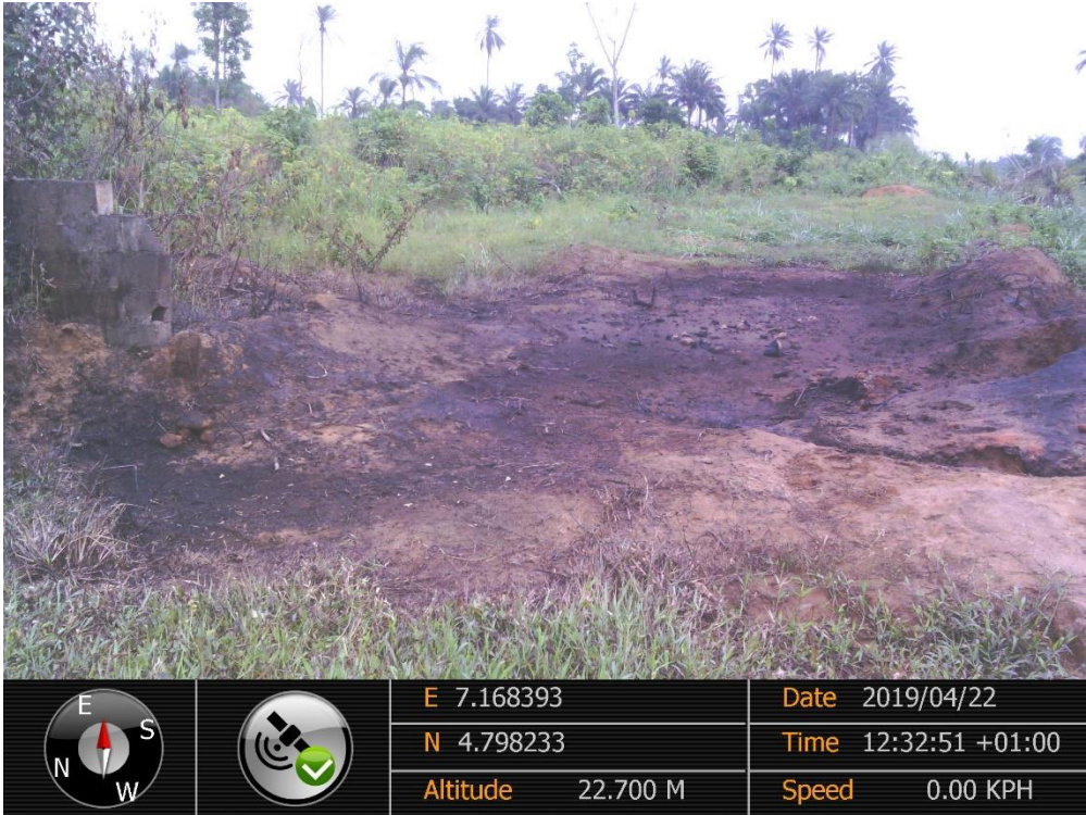
Overview: Part of spill impact on 24" Nkpoku – Bomu Pipeline Right of Way at Egbalor. Picture was taken during Joint Investigation of 22 nd April 2019.
