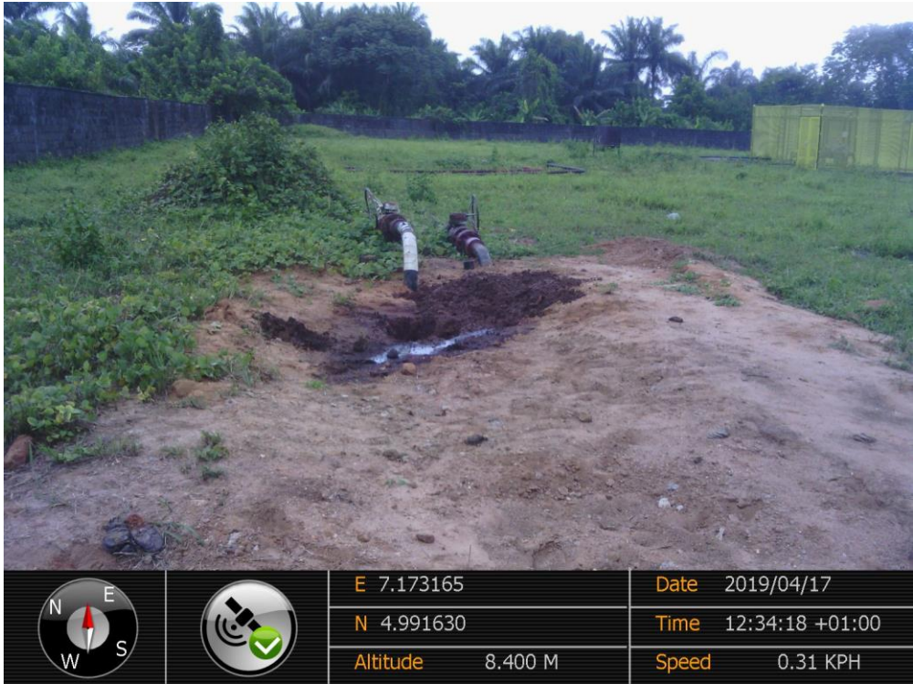
Overview: Part of spill impact on 4" Imo River2 Well 21L Flowline at Odagwa. Picture was taken during Joint Investigation of 17 th April 2019.
