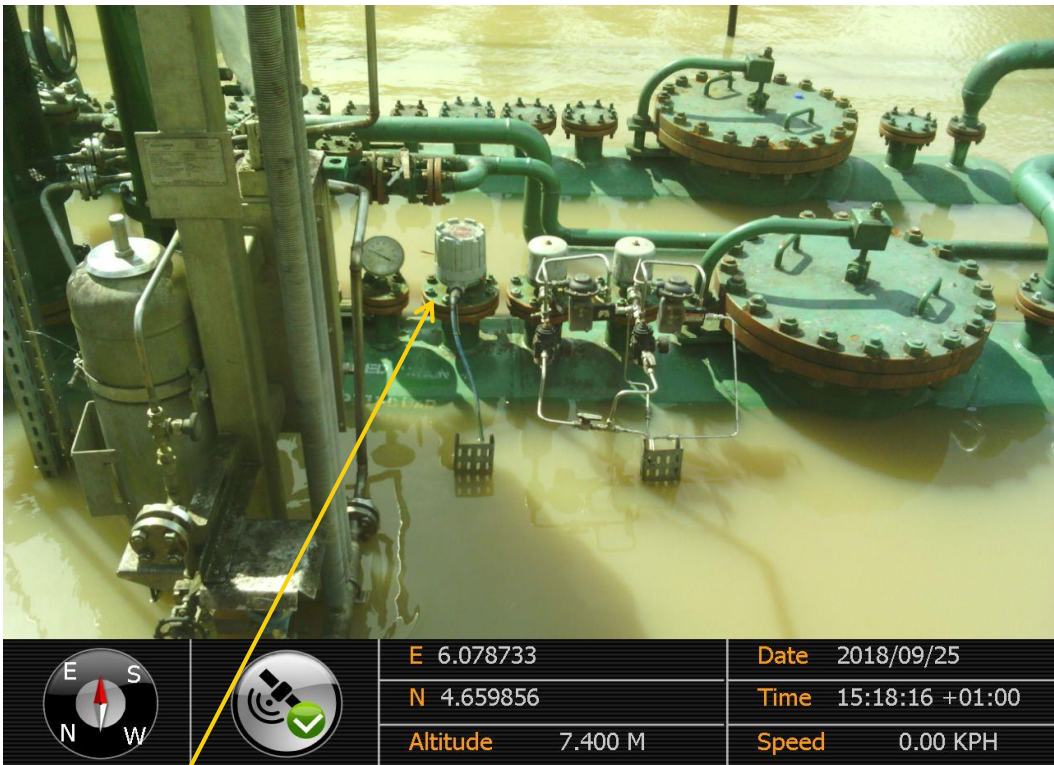
Close up: Failed Flange on 4" Diebu Creek Closed Drain Vessel Flange at Peremabiri. Picture was taken during Joint Investigation of 25 th September 2018.
