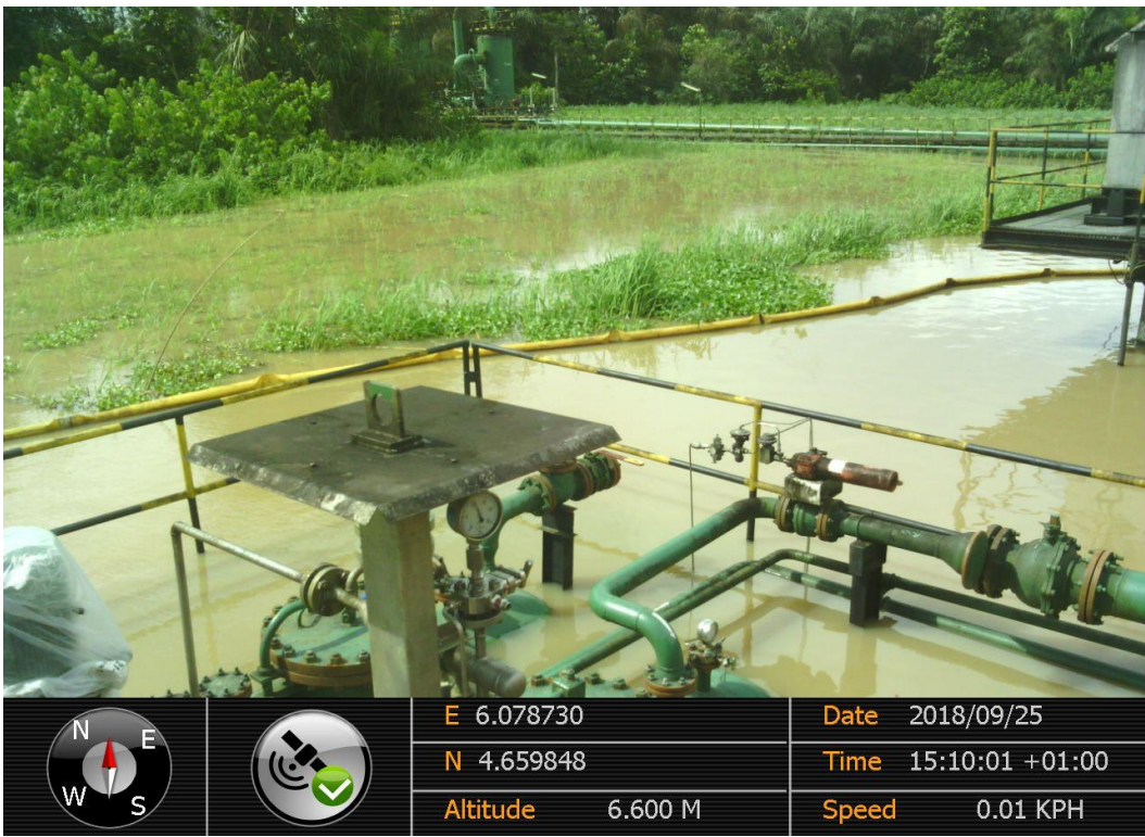
Overview: Part of spill impact on 4" Diebu Creek Closed Drain Vessel Flange at Peremabiri. Picture was taken during Joint Investigation of 25 th September 2018.
