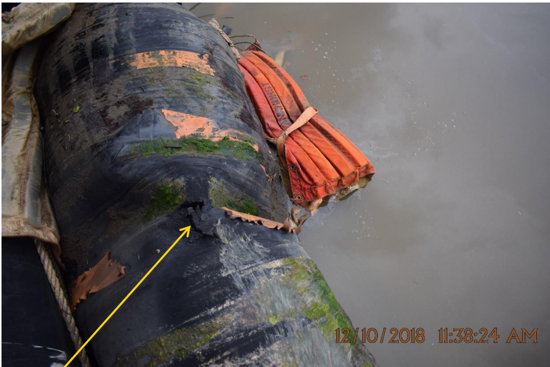
Close up: Laceration on Forcados Terminal Single Point Mooring2 (SPM2) at Ogulagha Kingdom. Picture was taken during Joint Investigation of 12th October 2018.
