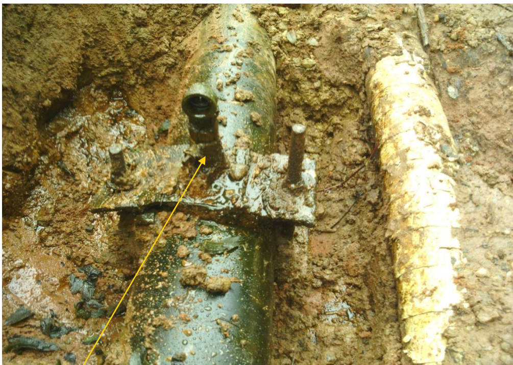
Close up: Illegal fitting on Imo River2 – Well 31L Flowline at Odagwa-Umuadeokwara . Picture was taken during Joint Investigation of 6 th September 2018.
