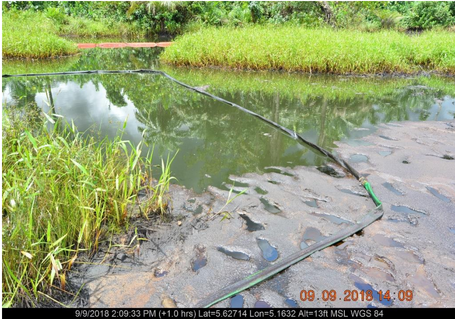
Overview: Part of spill impact on 20'' Otumara-Escravos Pipeline Right of Way at Ugboegungun. Picture was taken during Joint Investigation of 9 th September 2018.
