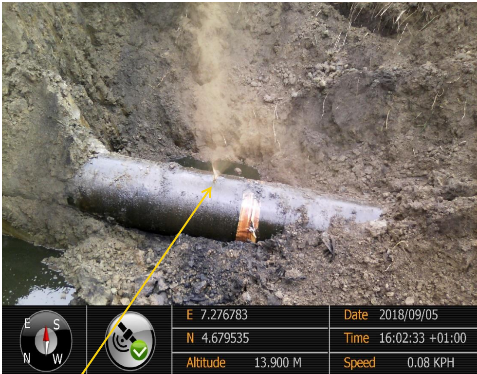
Close-up: Drilled Hole on 24" Nkpoku-Bomu Pipeline at Bera. Picture was taken during Joint Investigation of 5 th September 2018.
