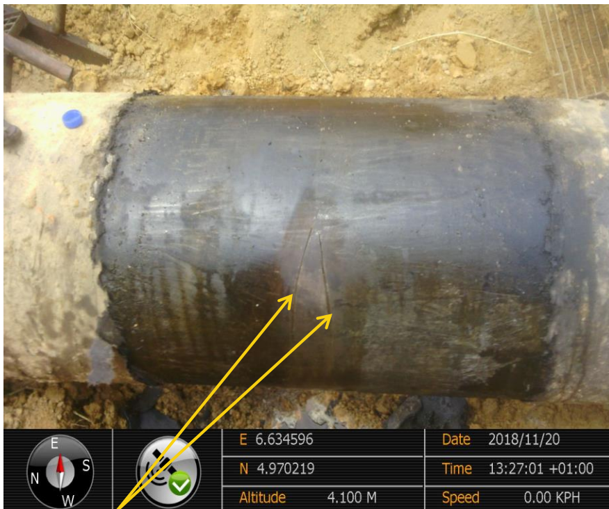
Close-up: Hacksaw Cuts on 20" Kolocreek - Rumuekpe Pipeline Right of Way at Okporowo. Picture was taken during Joint Investigation of 20 th November 2018.
