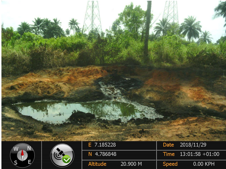
Overview: Part of spill impact on 24" Nkpoku - Bomu Pipeline Right of Way at Egbalor. Picture was taken during Joint Investigation of 29 th November 2018.
