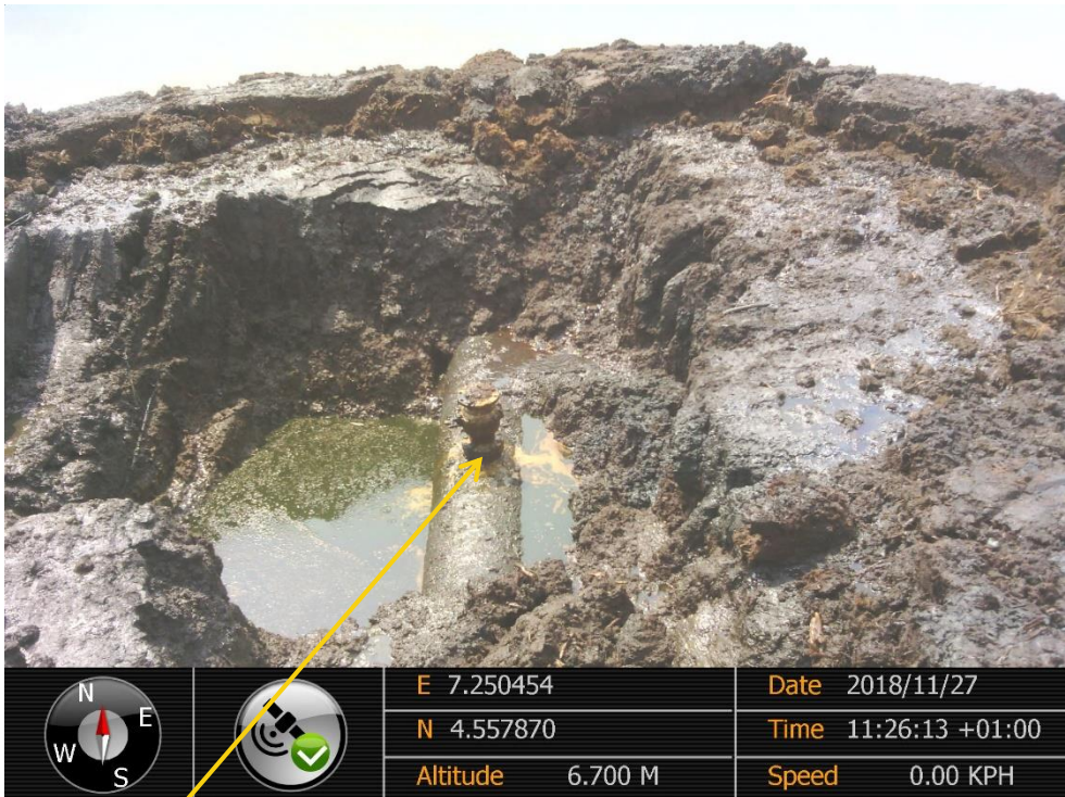
Close-up: Illegal fitting on 28" Bomu - Bonny Pipeline at Owokiri. Picture was taken during Joint Investigation of 27 th November 2018.
