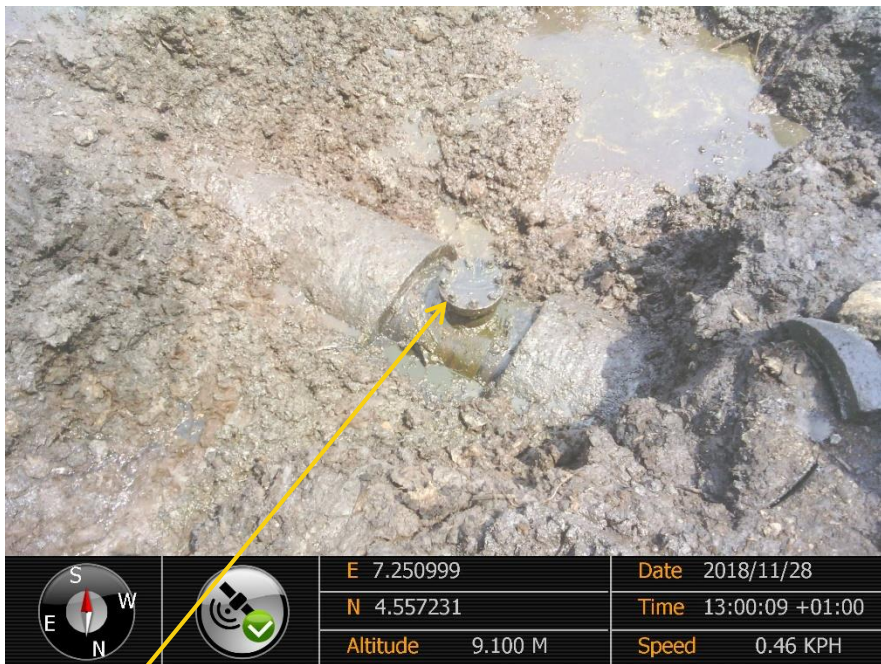
Close-up: Illegal fitting on 24" Bomu-Bonny Pipeline at Owokiri. Picture was taken during Joint Investigation of 28 th November 2018.
