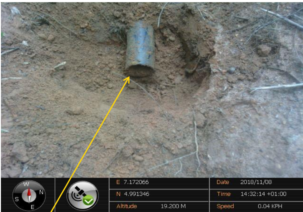
Close-up: Section of Missing Flowline on 4" Imo River 2 Well 21S Flowline at Odagwa. Picture was taken during Joint Investigation of 8 th November 2018
