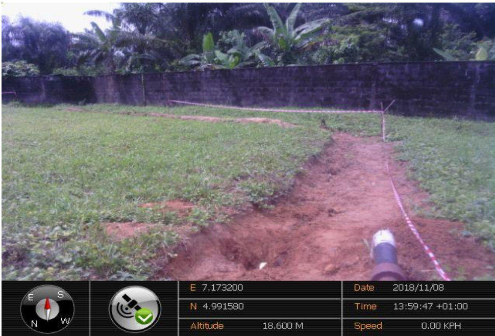
Overview: Part of spill impact on 4" Imo River 2 Well 21S Flowline at Odagwa. Picture was taken during Joint Investigation of 8 th November 2018.
