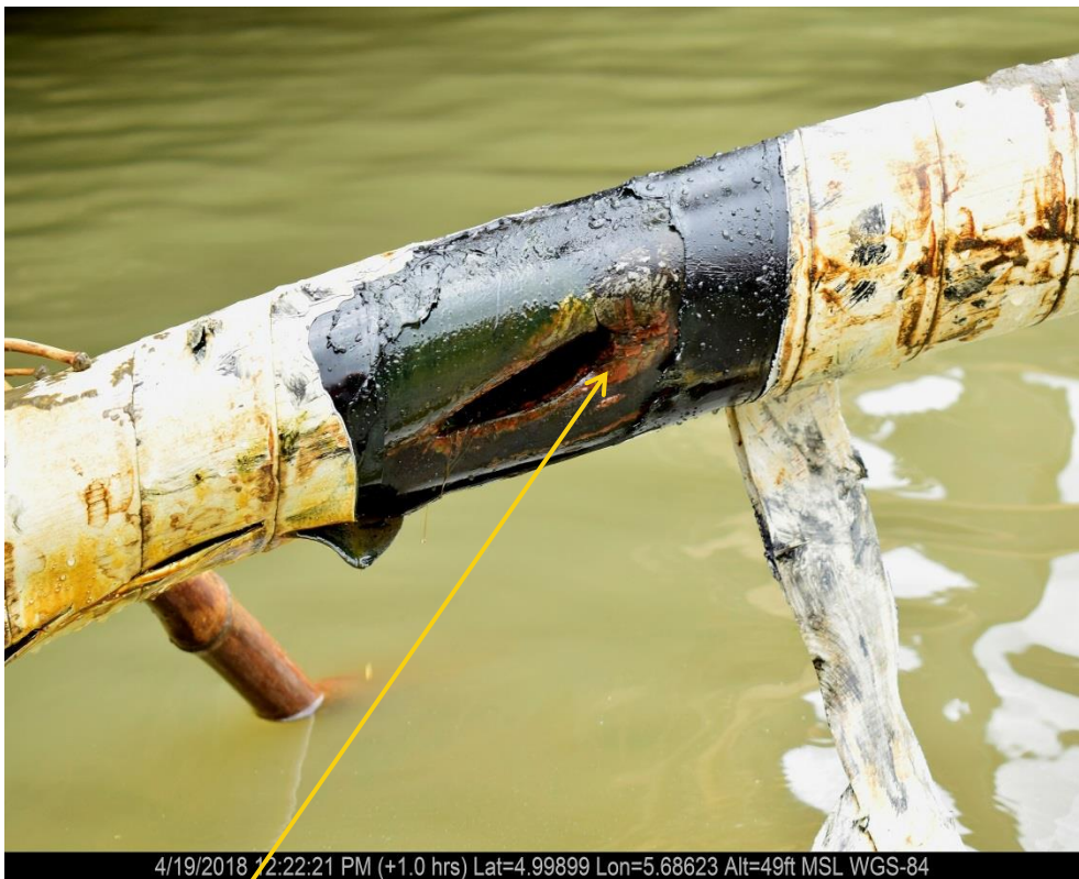
Close-up: Inward Dent & Tear on Benisede Well-5T Flowline at Ojobo. Picture was taken during Joint Investigation of 19 th April 2018.
