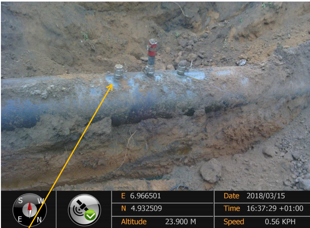
Close-up: One of three Illegal fittings on 20''Rumuekpe-Nkpoku Pipeline at Mbodo-Aluu. (The other two were non-leaking).
