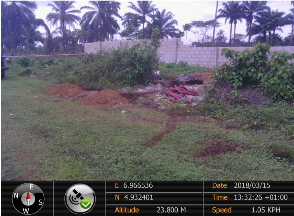
Overview: Part of spill impact on 20''Rumuekpe-Nkpoku Pipeline Right of Way at Mbodo-Aluu. Picture was taken during Joint Investigation of 15 th March 2018.
