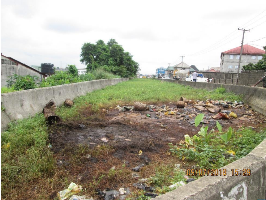
Overview: Part of spill impact on 28" Nkpoku - Bomu Pipeline at Rumuokwurusi. Picture was taken during Joint Investigation of 9 th July 2018.
