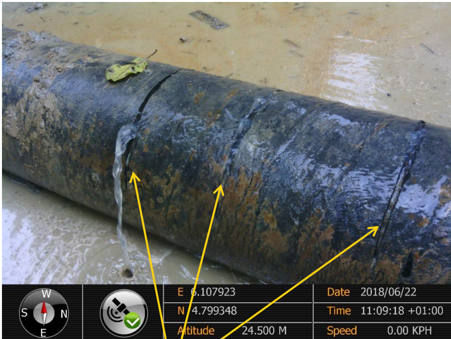
Close-up: Multiple Leaking Hacksaw Cuts on 10" Diebucreek-Nunriver Pipeline at Oporoma. Picture was taken during Joint Investigation of 22 nd June 2018.
