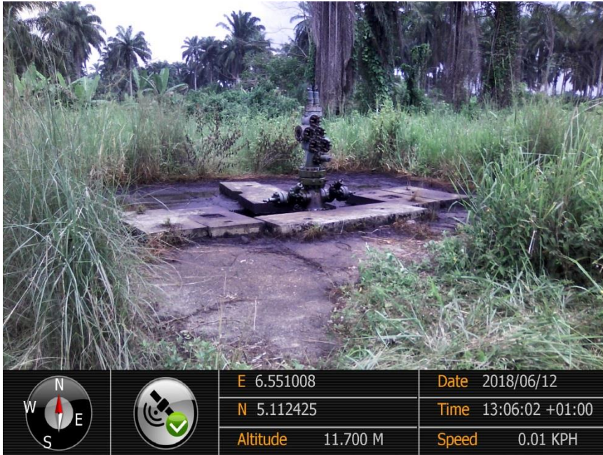
Overview: Part of spill impact Ubie Well 5 L/S Well head at Idu-Ekpeye. Picture was taken during Joint Investigation of 12 th June 2018.
