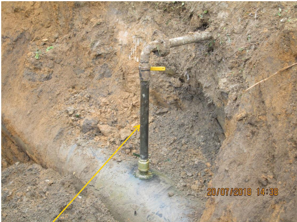
Close-up: Illegal fitting on 20" Rumuekpe-Nkpoku Pipeline at Mbodo-Aluu. Picture was taken during Post Joint Investigation of 20 th July 2018.
