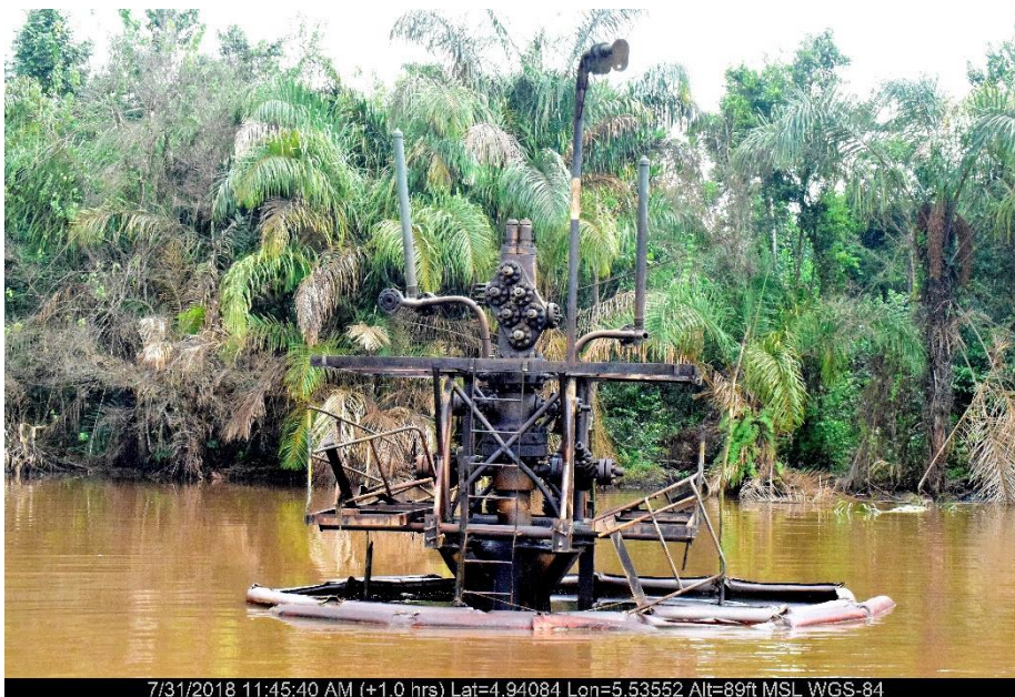
Overview: Part of spill impact on Agbaya well-1 Wellhead at Ogbotobo-Agbayama. Picture was taken during Joint Investigation of 31 st July 2018.
