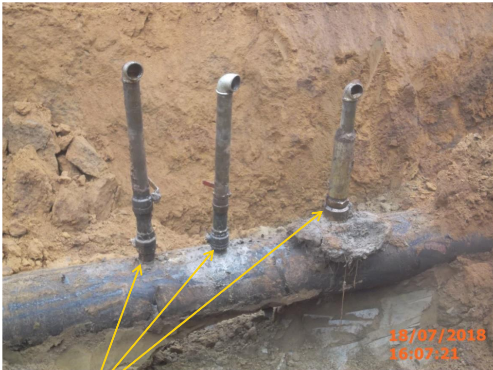
Close-up: Illegal Fittings on 12" Imo River-Ogale Pipeline at Umuololo-Etitiuzo. Picture was taken during Joint Investigation of 18 th July 2018.
