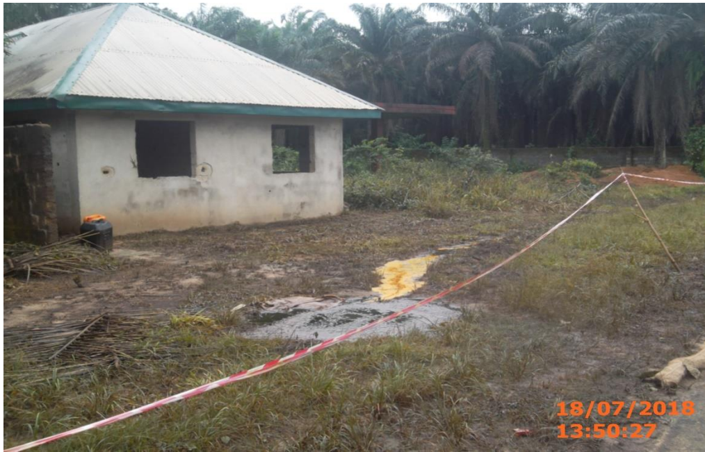
Overview: Part of spill impact on 12" Imo River-Ogale Pipeline Right of Way at Umuololo-Etitiuzo. Picture was taken during Joint Investigation of 18 th July 2018.
