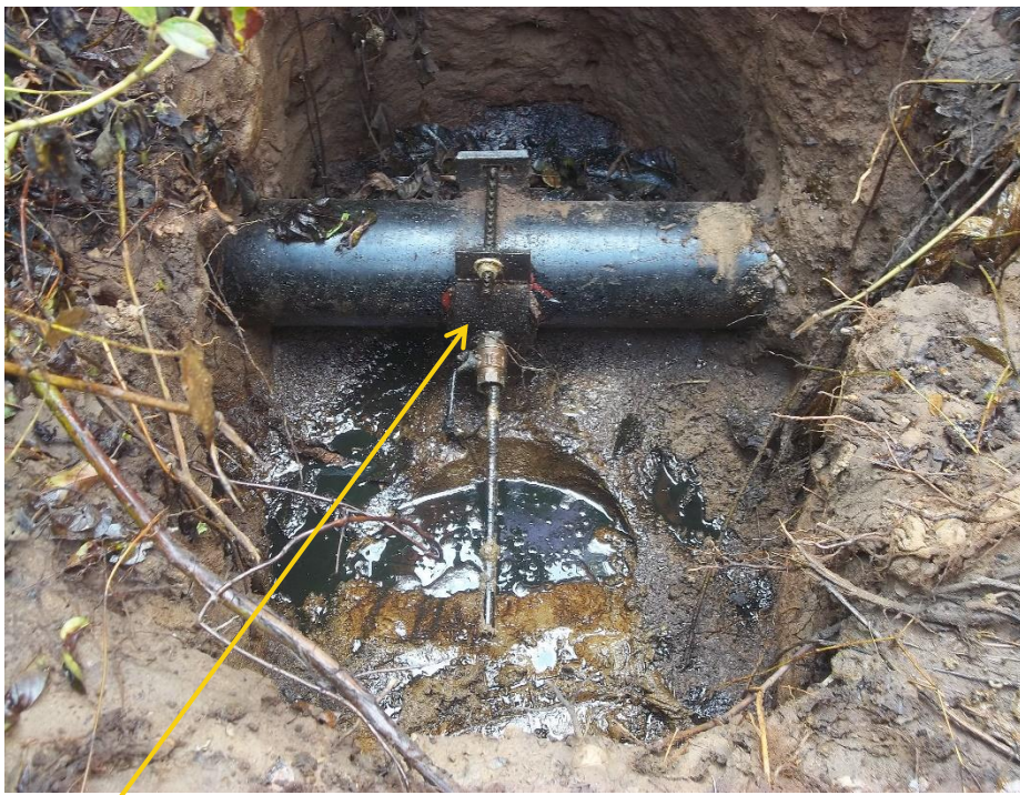
Close-up: Illegal fitting on Imo River Well59 Flowline at Igiriukwu. Picture was taken during Joint Investigation of 10 th July 2018.
