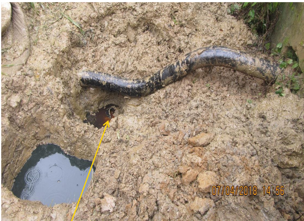
Close-up: Leaking Disused 6" Kolocreek Well-19T Flowline at Imiringi. Picture was taken during Joint Investigation of 4th July 2018.
