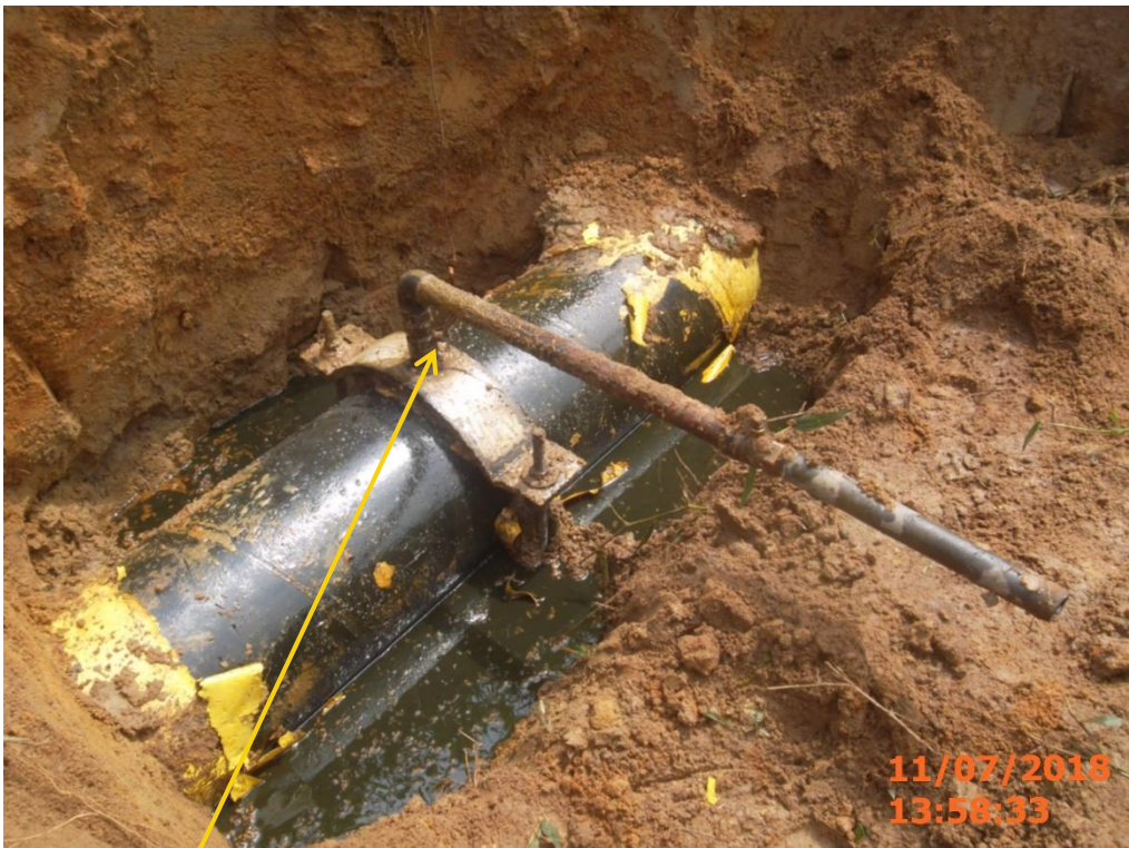
Close-up: Illegal fitting on 12" Imo Rive2-Ogale Pipeline at Igiriukwu-Isi-Etithoha Picture was taken during Joint Investigation of 11 th July 2018.
