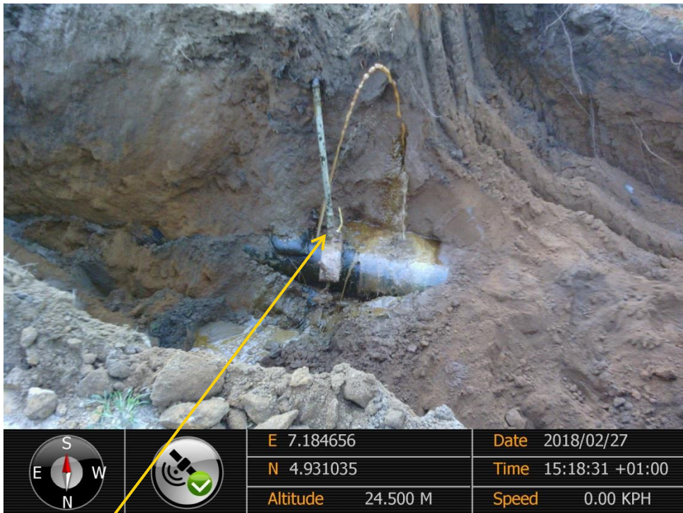
Close-up: Illegal fitting on 12" Imo River – Ogale Pipeline at Okohia. Picture was taken during Joint Investigation of 27 th February 2018.
