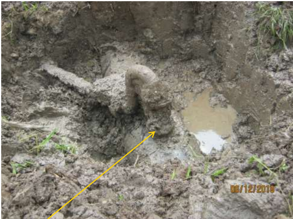
Close-up: Illegal fitting on 20" Kolocreek-Rumuekpe Pipeline at Imogu-Rumuekpe. Picture was taken during Joint Investigation of 12 th June 2018.
