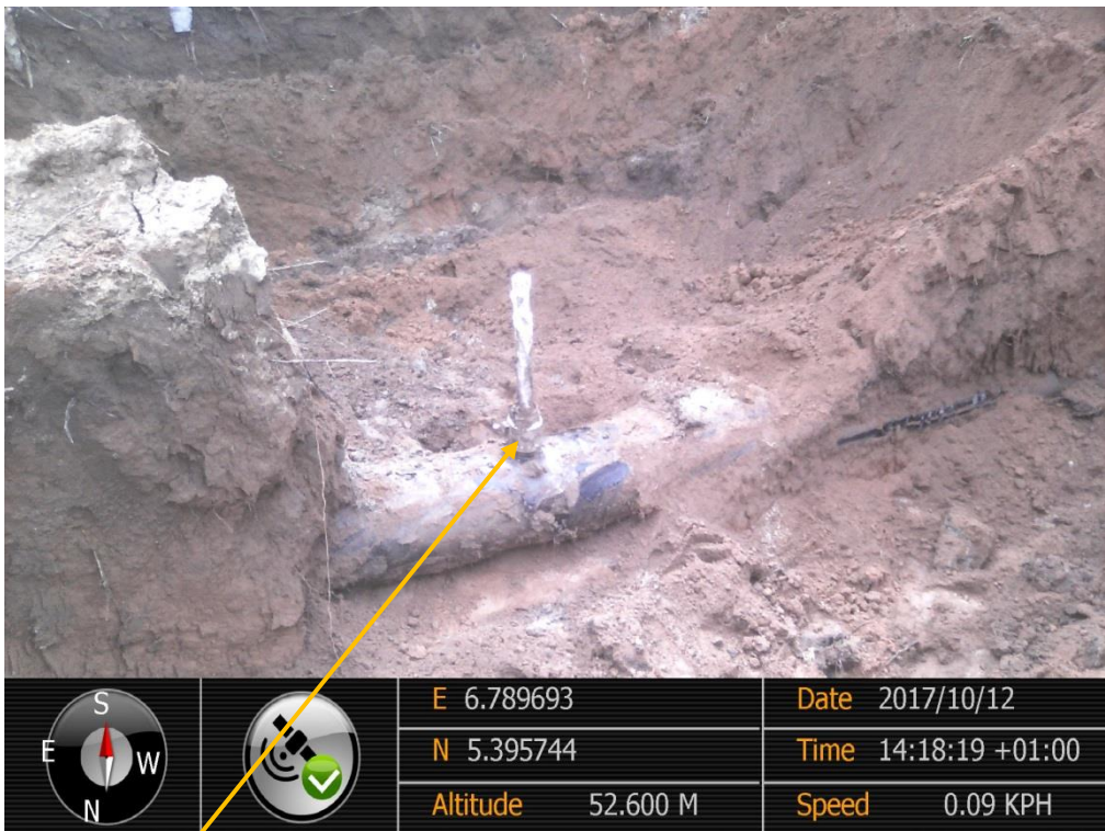
Close-up: Illegal fitting on 16" Egbema-Assa Pipeline at Obile. Picture was taken during Joint Investigation of 12 th October 2017.
