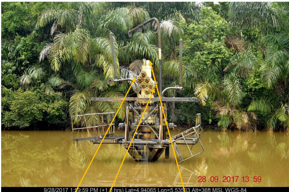
Close-up: Position of Stolen CCU, Bean Box and Wellhead Survey Cap on Agbaya well 1 Wellhead at Agbayama. Picture was taken during Joint Investigation of 28 th September 2017.
