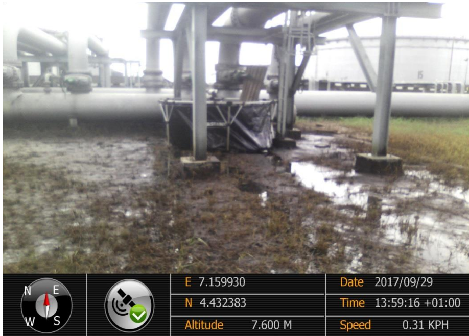
Overview: Part of spill impact 01 MOV-411 Filling Valve Flange to Tank 2 at Bonny Terminals. Picture was taken during Joint Investigation of 29 th September 2017.
