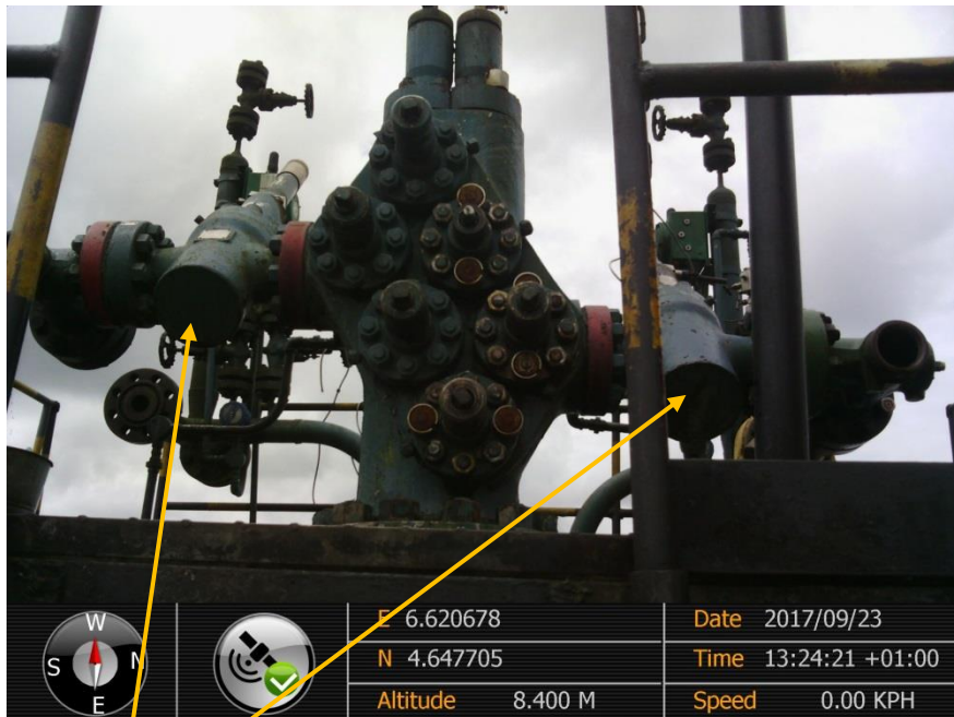
Close-up: Position of Removed Bean Box cover on Soku Well 22 Well Head. Picture was taken during Joint Investigation of 23 rd September 2017.
