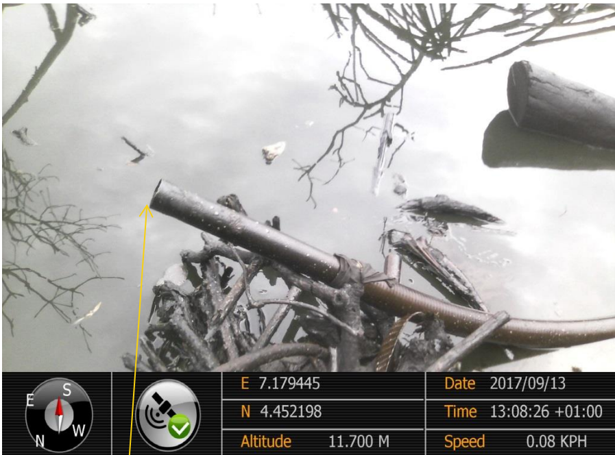
Close-up: Leak point on 28" Bomu-Bonny Pipeline at Ogbonga Forest Oloma. Picture was taken during Joint Investigation of 13 th September 2017.
