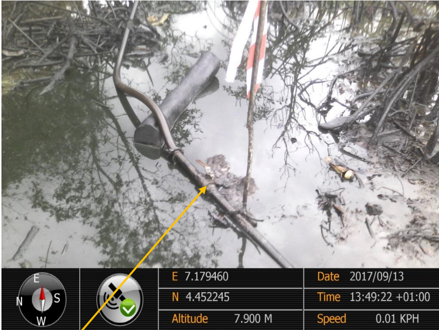
Close-up: Illegal pipe and failed 2" ball valve hose connection on 28" Bomu-Bonny Trans Niger Pipeline at Ogbonga Forest Oloma. Picture was taken during Joint Investigation of 13 th September 2017.
