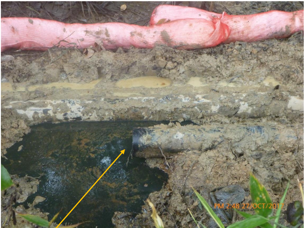
Close-up: Missing Flowline on 4" Adibawa Well 23 Disused Flowline at Edagberi Better Land. Picture was taken during Joint Investigation of 27 th October 2017.
