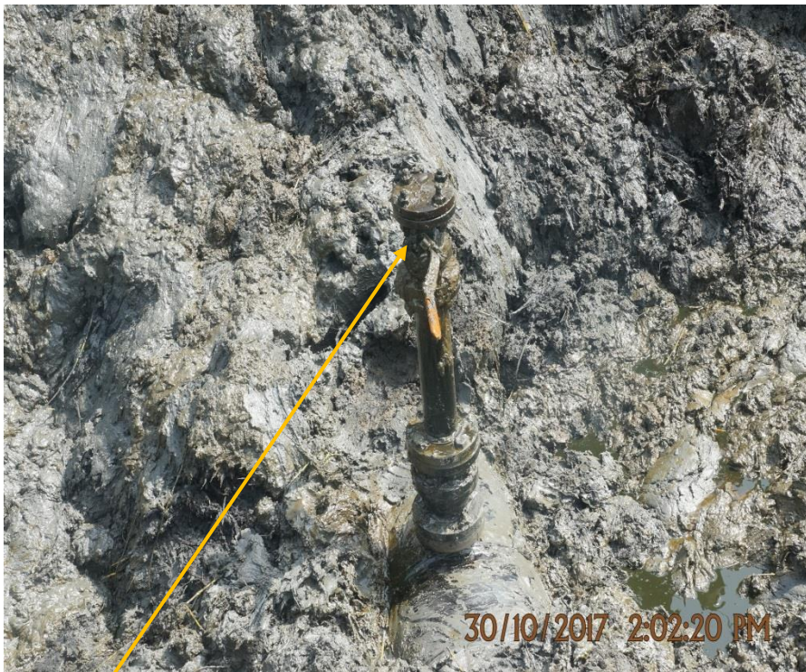
Close-up: Illegal fitting on 20" Otumara-Escravos Pipeline at Ugboegungun. Picture was taken during Joint Investigation of 30 th October 2017.
