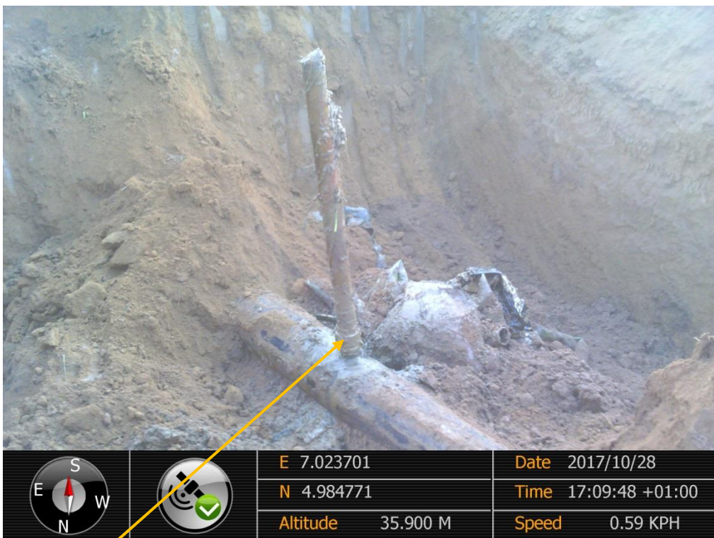
Close-up: Illegal fitting on 8" Umuechem - Nkpoku pipeline at Omunwei. Picture was taken during Joint Investigation of 28 th October 2017.
