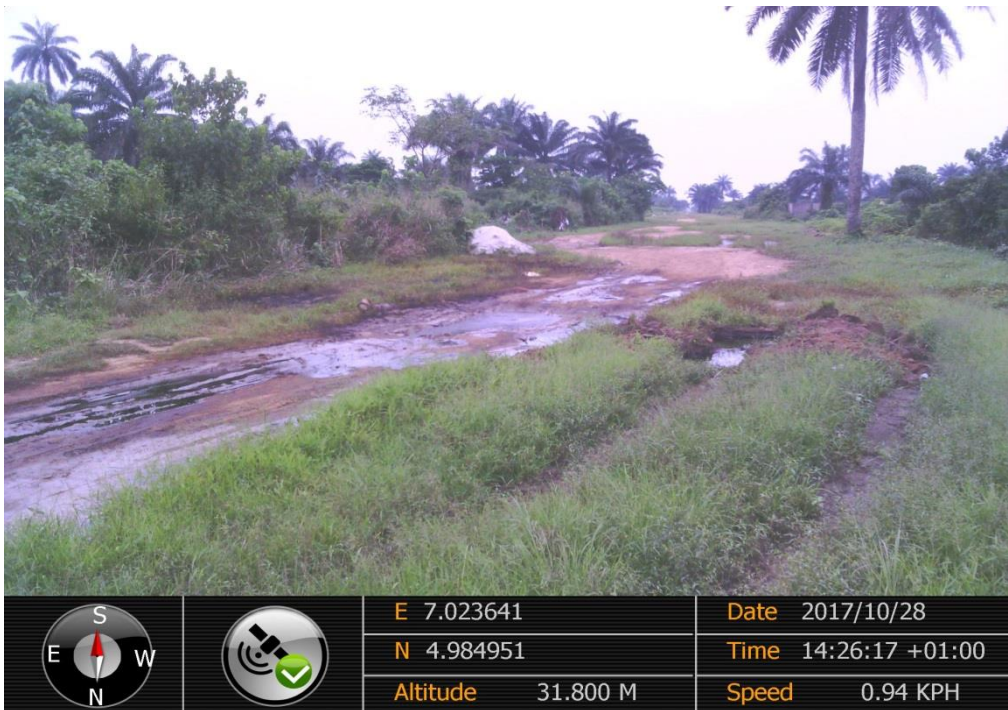
Overview: Part of spill impact on 8" Umuechem - Nkpoku pipeline at Omunwei. Picture was taken during Joint Investigation of 28 th October 2017.
