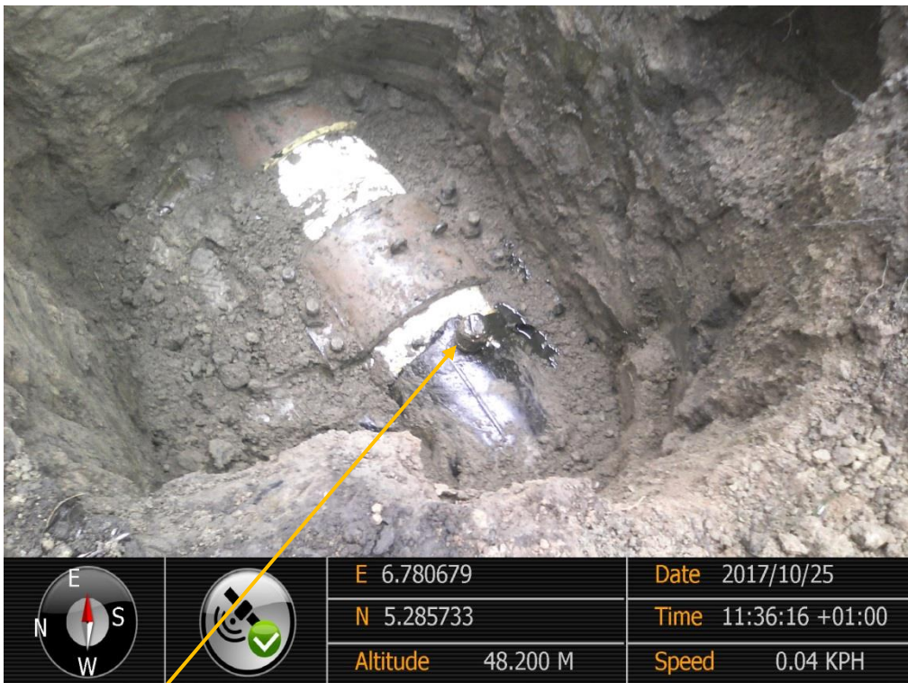
Close-up: Illegal fitting on 18" Assa-Rumuekpe Pipeline at Awara. Picture was taken during Joint Investigation of 25 th October 2017.
