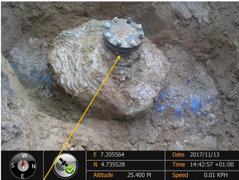
Close-up: Illegal Fitting on 28" Nkpoku-Bomu Pipeline at Norkpo. Picture was taken during the Initial Site Visit of 13 th Nov. 2017.
