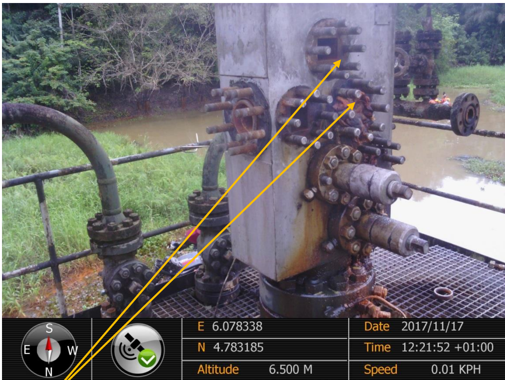
Close-up: Position of Missing Survey Valves on Nun River Well 15 Wellhead at Onyoma. Picture was taken during Joint Investigation of 17 th November 2017.
