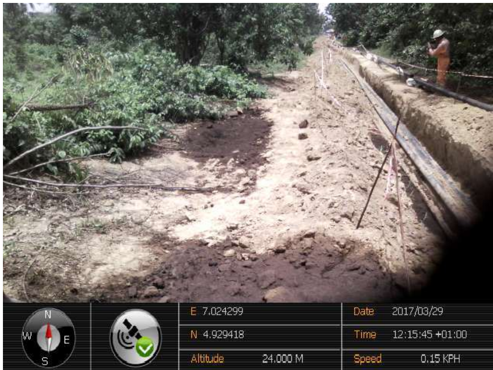
Overview: Part of spill impact on Agbada 2 Well34S 4" Flowline Right of Way at Omueke . Picture was taken during initial site visit on 29 th March 2017.
