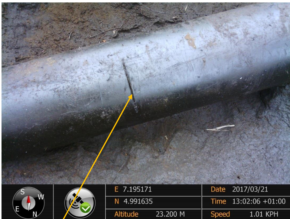
Close-up: Hacksaw cut on 6" Imo River 3 Well 37L Flowline at Igiriukwu-Owaza. Picture was taken during Joint Investigation of 21 st March 2017.
