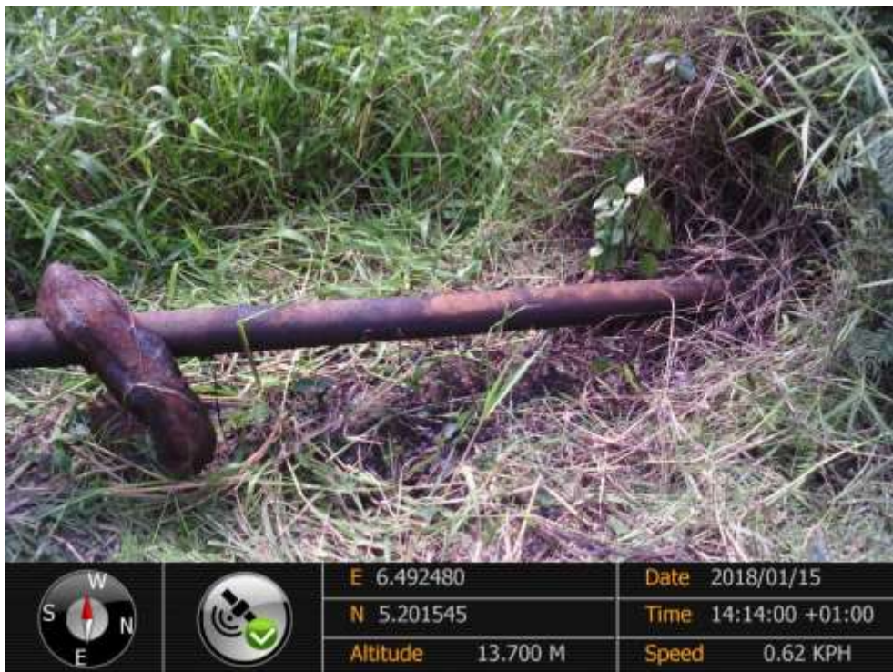
Close-up: No spill point found on 4" Adibawa Well 4 & 7 flowline at Edagberi. Picture was taken during Joint Investigation of 15 th January 2018.
